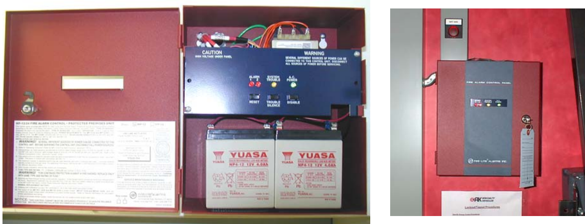
Figure 21: Fire Alarm Control Panel
