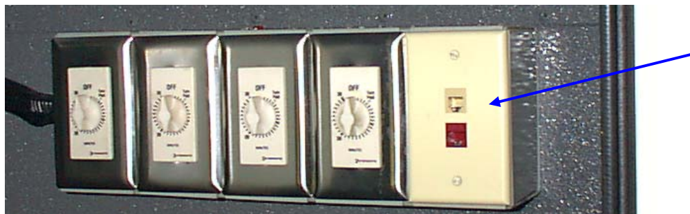
Figure 13: Phone & Data Line Connections
