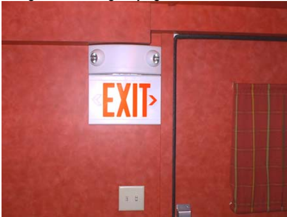
Exhibition Kitchen Emergency Light
