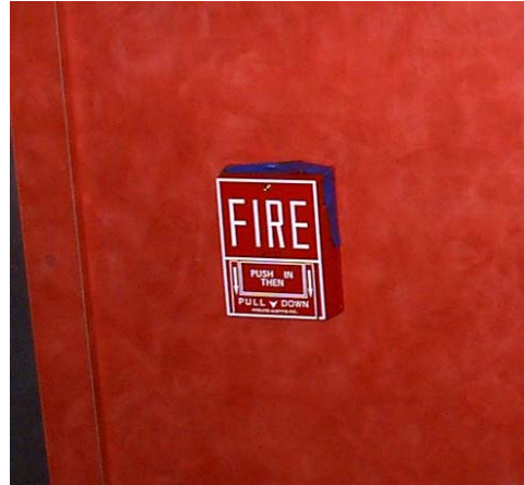
Figure 22: Fire Alarm Pull Station
