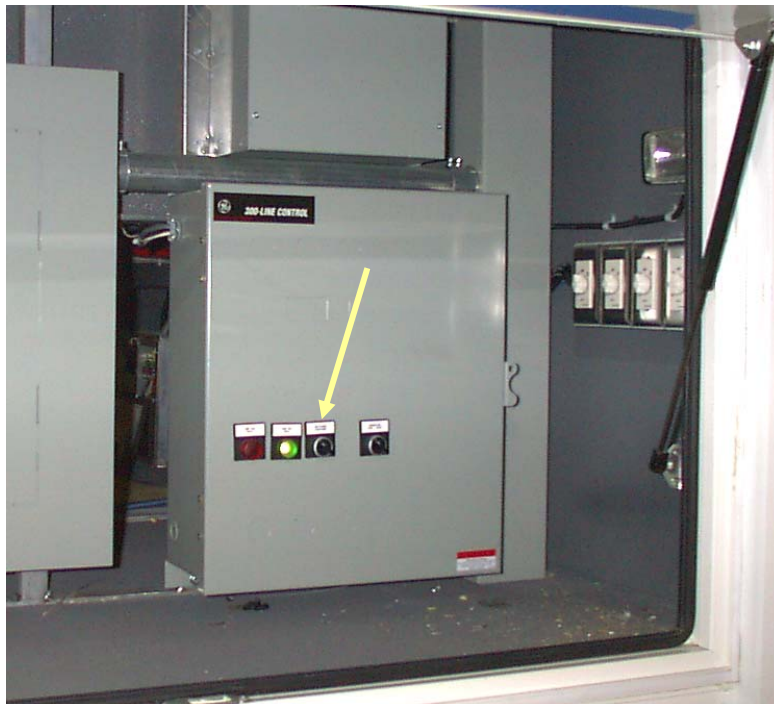
Figure 23: Line/Off/Generator (LOG) Switch
