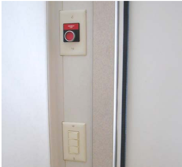
Emergency Off button, Control Room, next to Entry Door
