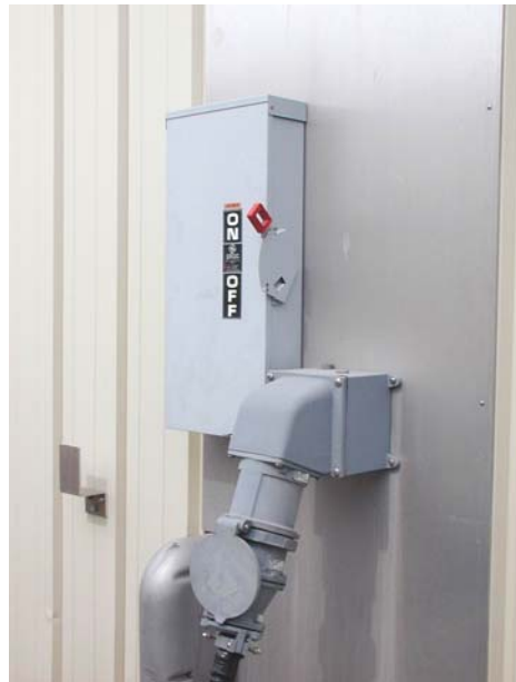
Figure 38: Shore Power Connection
