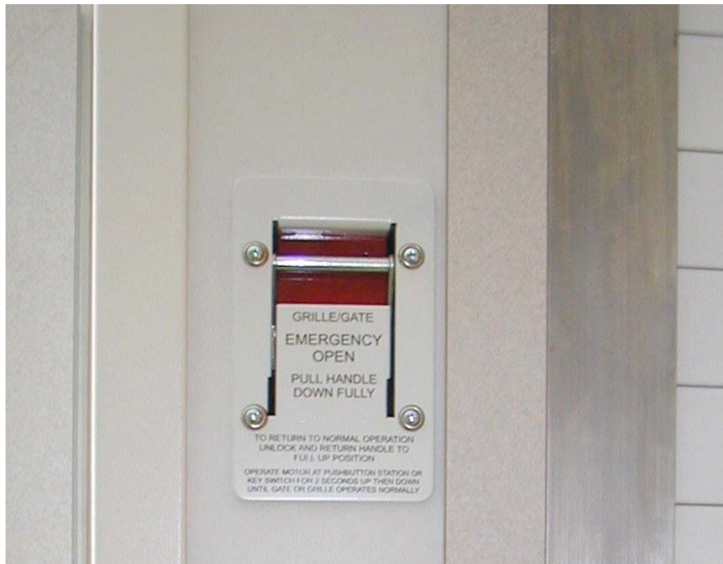
Figure 33: Roll Door Emergency Release
