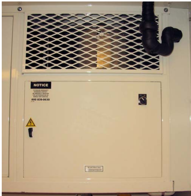
Figure 43: A/C / Chiller Control Panel
