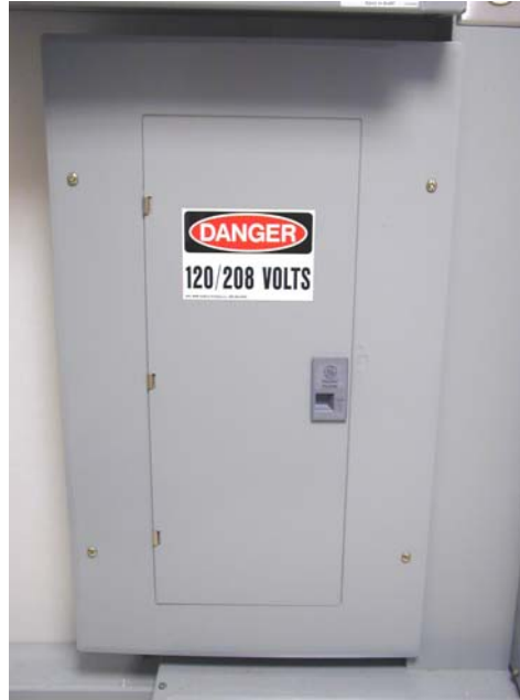
Figure 35: 120/208V AC Electrical Panel
