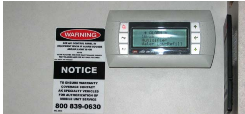
Figure 44: HVAC Monitor and Alarm Panel
