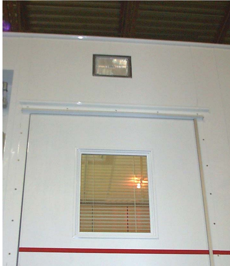
Figure 57: Staff Door Lighting
