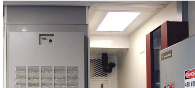
Figure 59: Equipment Room Lighting
