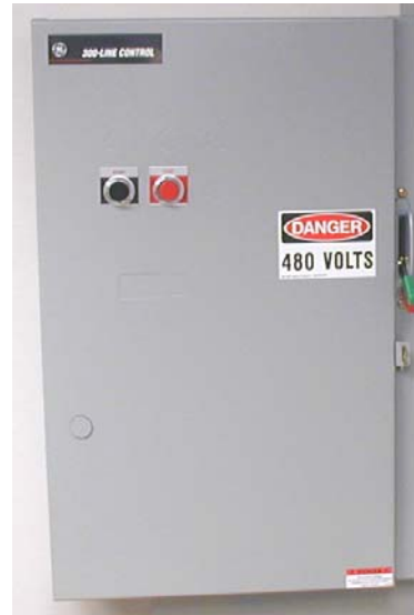
A1 Start/Stop in Equipment Room
