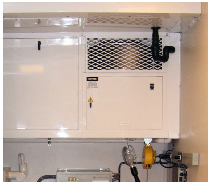
Figure 8: Equipment Room Overall
