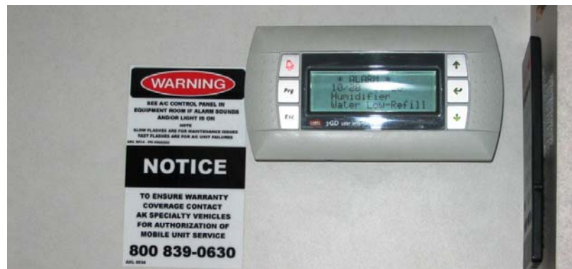
HVAC Monitor & Alarm
