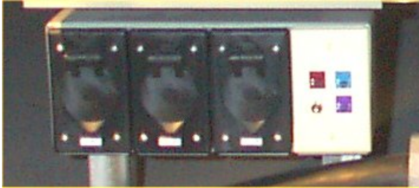
Figure 18: Phone & Data Line Connections
