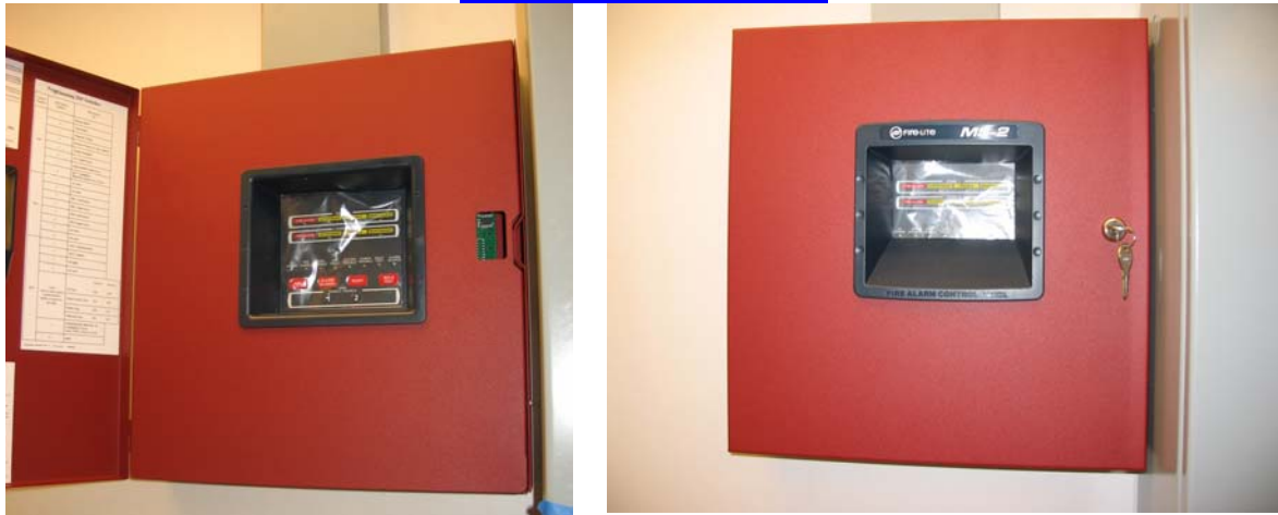
Figure 28: Fire Alarm Control Panel
