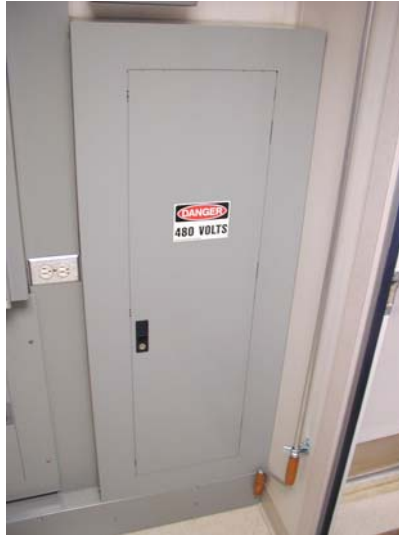
Figure 36: 480V AC Electrical Panel
