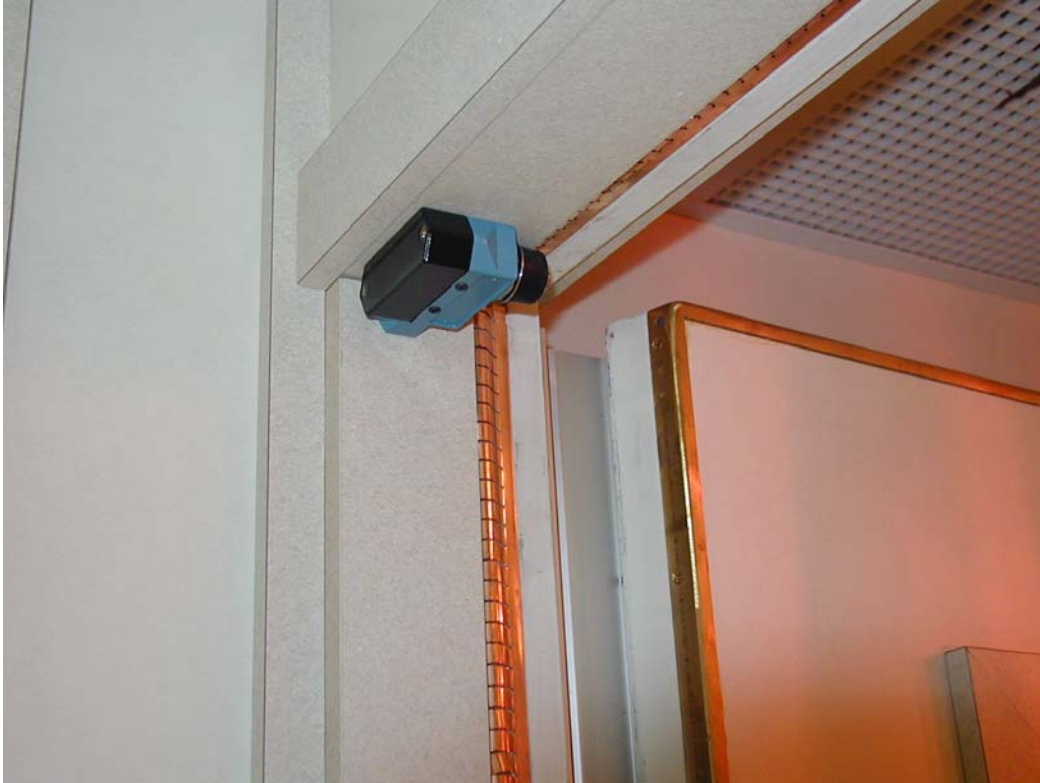
Close up of RF door trim
