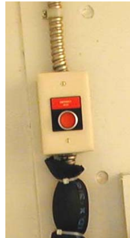
Emergency Off Button, Magnet Room
