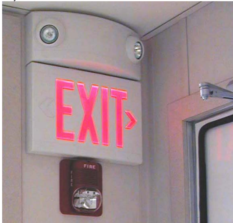
Figure 54: Emergency Dual Beam Lighting
