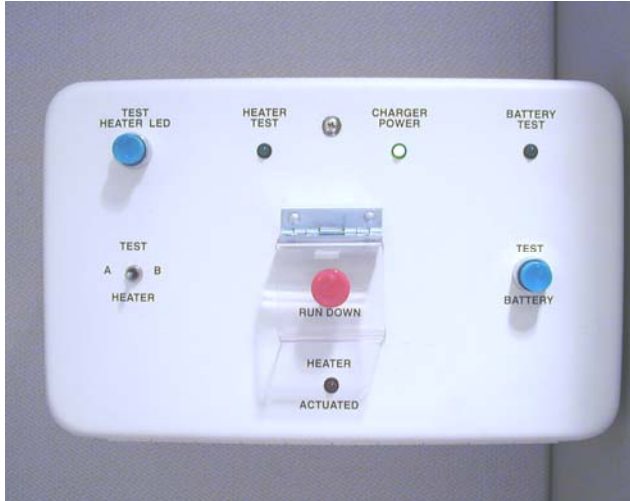
Guarded Magnet Quench Button, Scan Room
