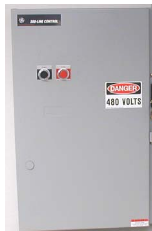
Figure 37: A1 Electrical Panel
