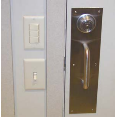
Scan Room and Magnet Room Lighting
