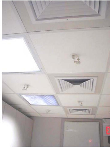
Figure 60: Control Room Lighting
