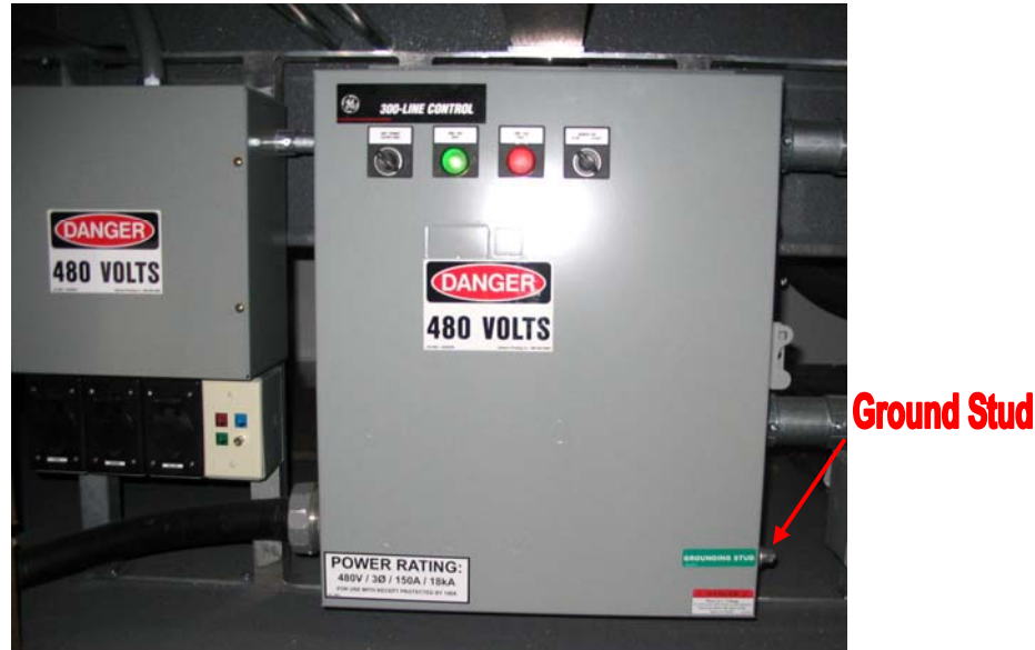
Figure 40: Power Supply Control Panel Ground Connection
