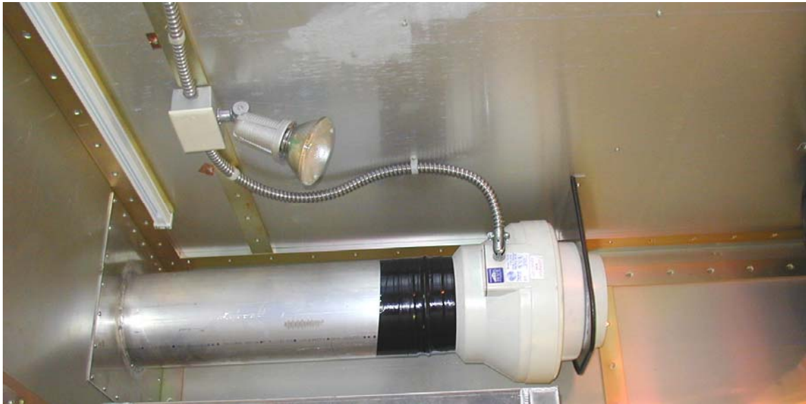
Figure 16: Magnet Room Helium Gas Exhaust Fan
