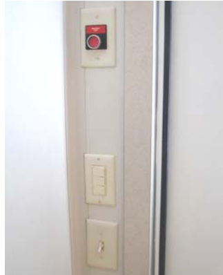
Control Room and Equipment Room Lighting and E-Stop Controls
