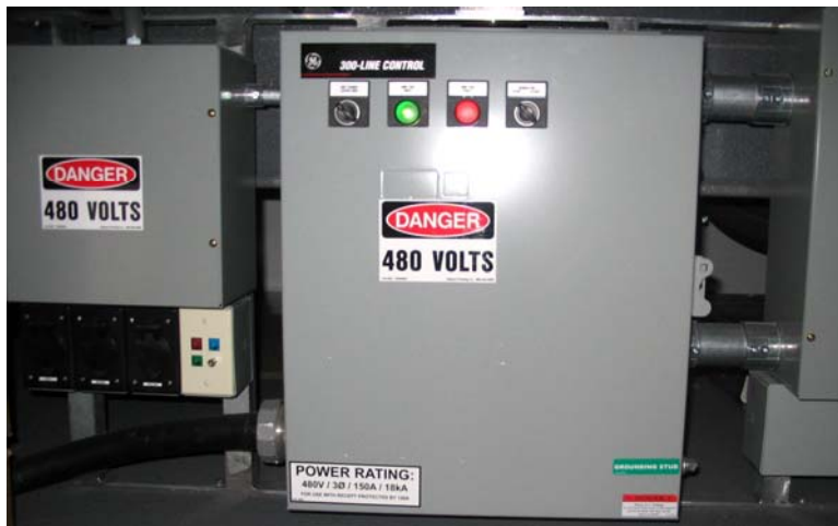
Figure 11: Power Supply Control Panel
