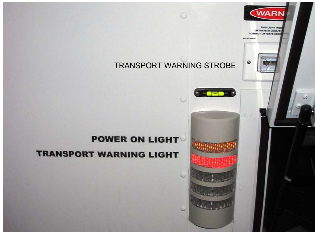
Figure 64: Lift Transport Warning Strobe
