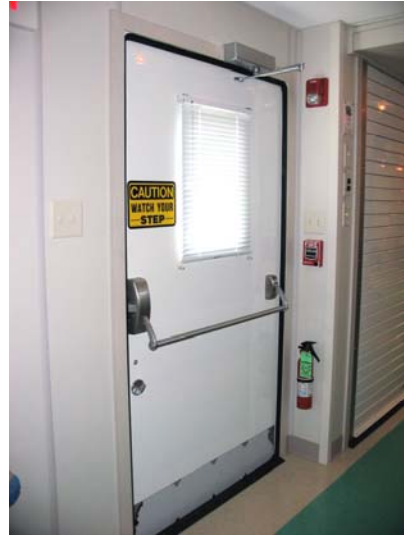
Staff Entry Door Controls
