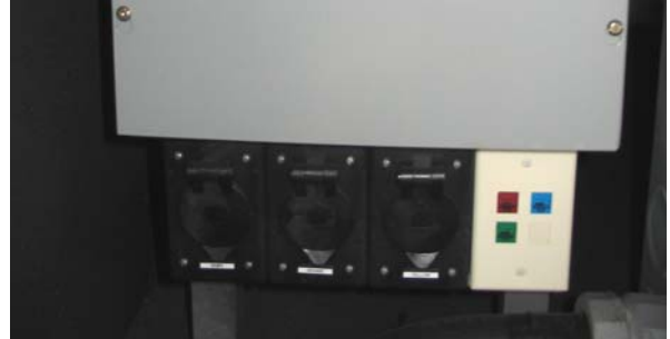
Figure 13: Phone & Data Line Connections
