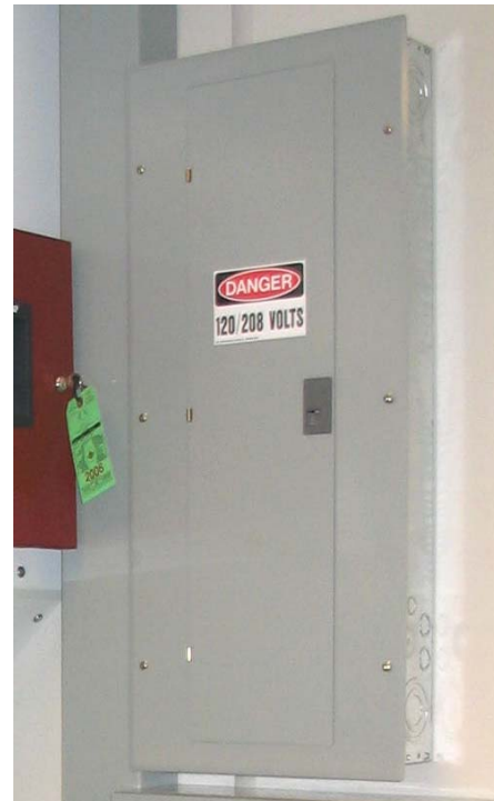
Figure 25: 120/208V AC Electrical Panel (interior)
