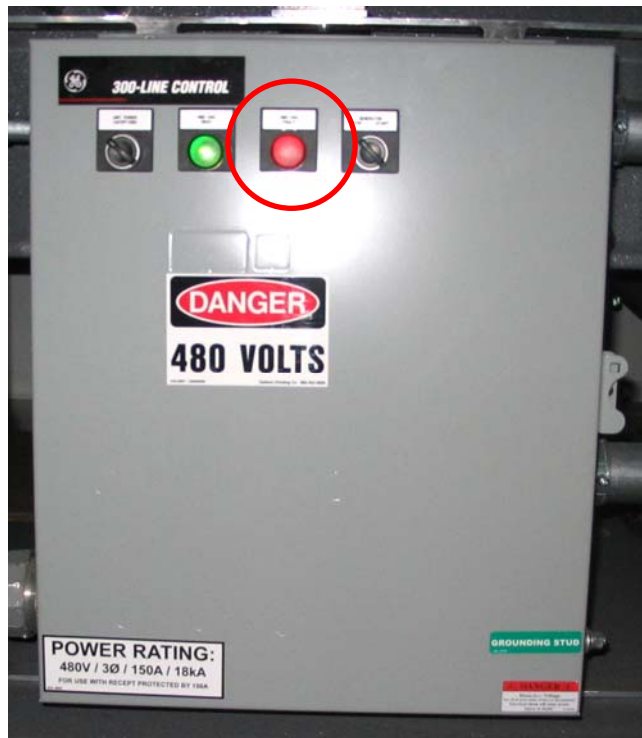
Figure 48: 480V AC Fault Indicator Light
