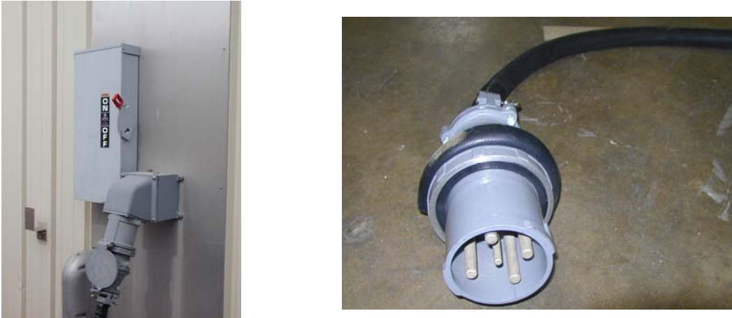
Figure 26: Shore Power Connection
