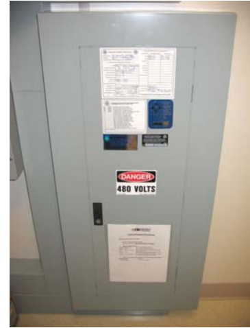
Figure 24: 480V AC Electrical Panel (interior)
