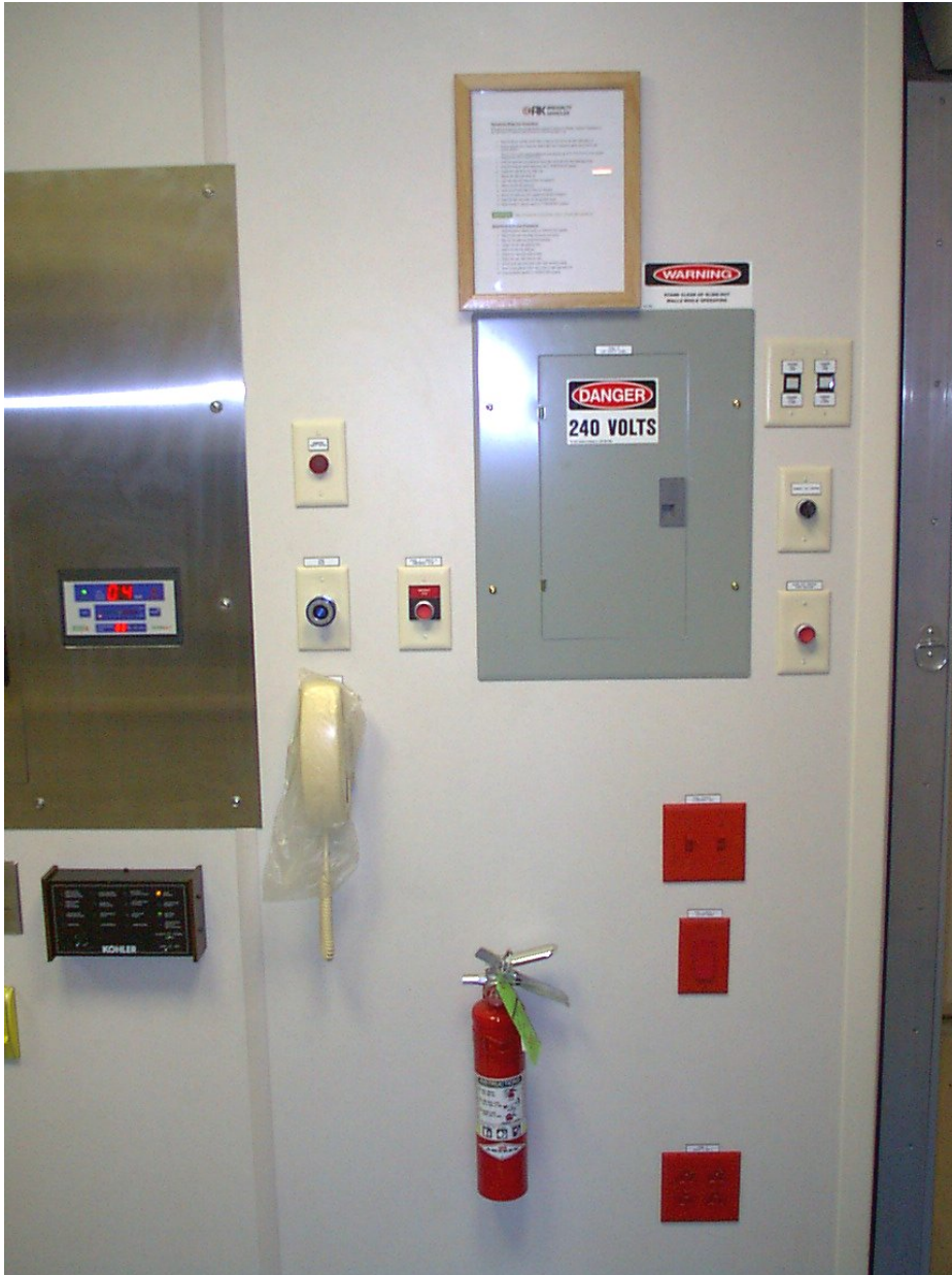
Figure 11: Procedure Room Controls
