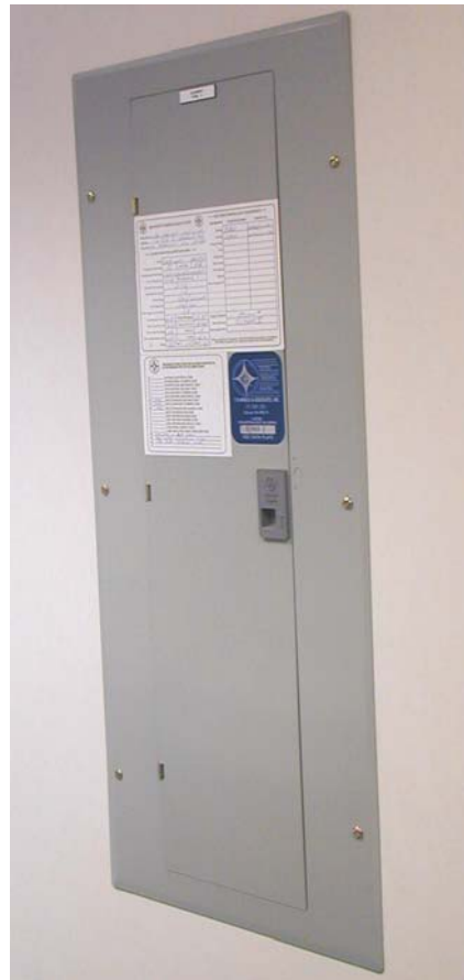
Control Room Panel
