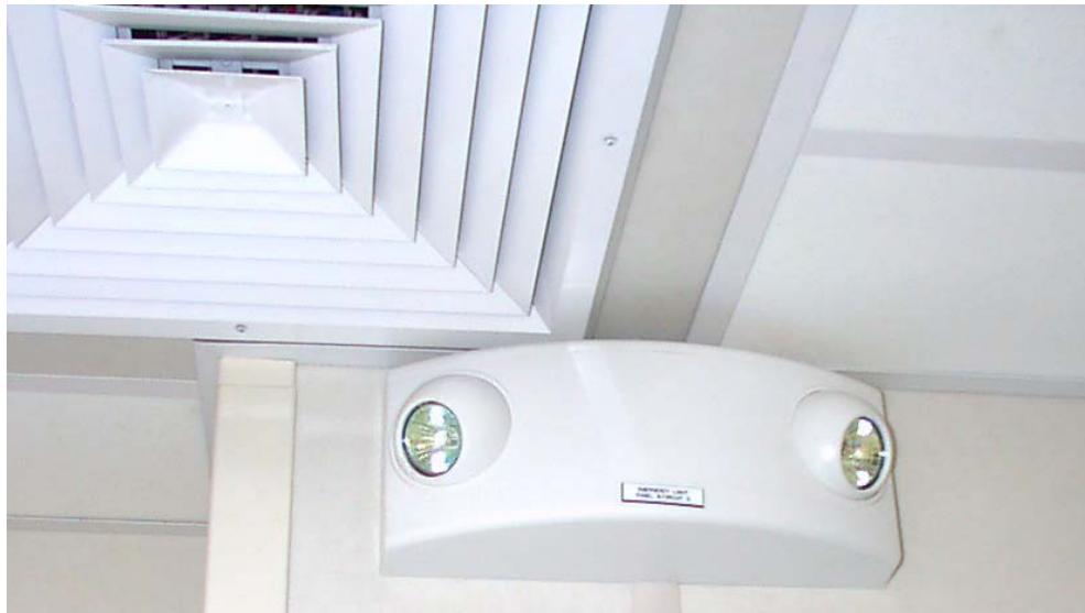
Figure 58: Emergency Dual Beam Lighting (Typical)
