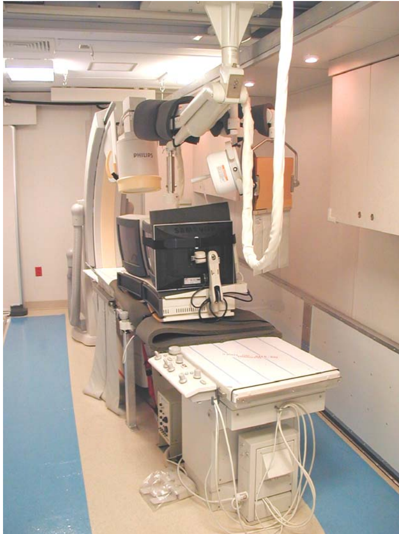
Figure 12: Procedure Room Equipment (Secured for Transport)
