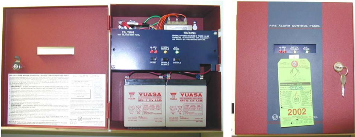
Figure 32: Fire Alarm Control Panel
