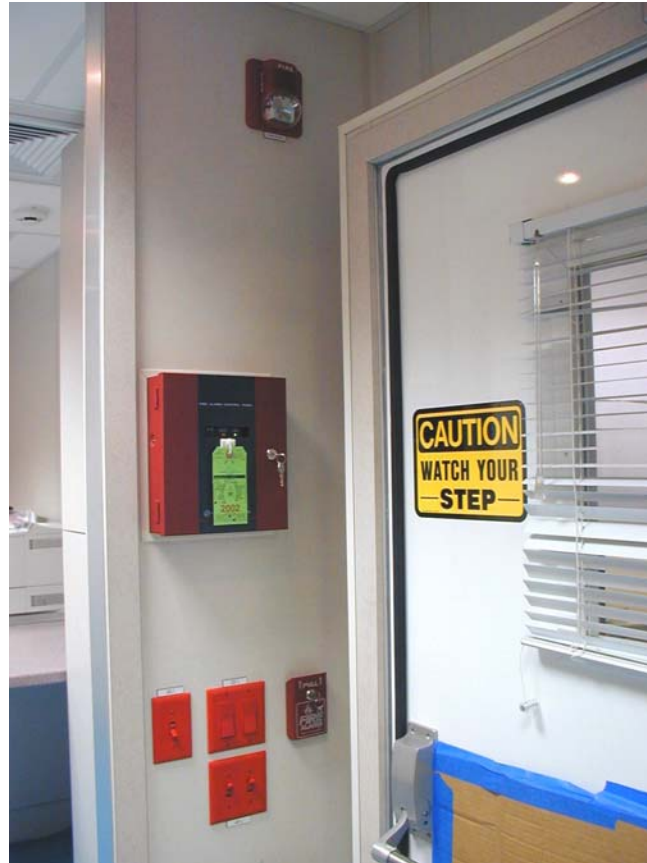
Figure 10: Control Room Controls
