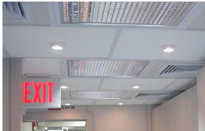
Figure 62: Control Room Lighting
