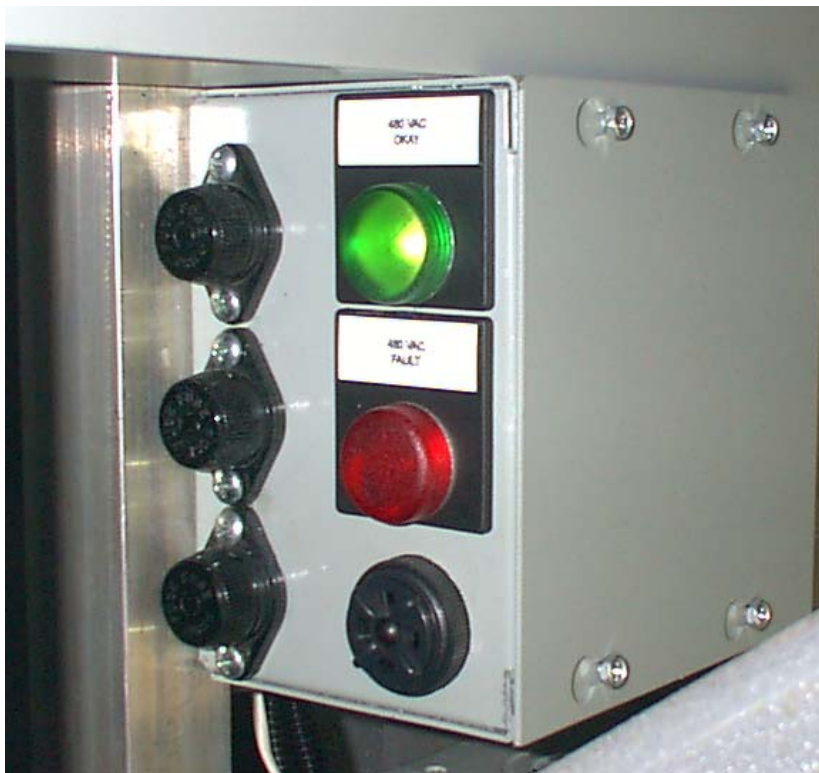
Figure 47: 480V AC Phase Power Monitor
