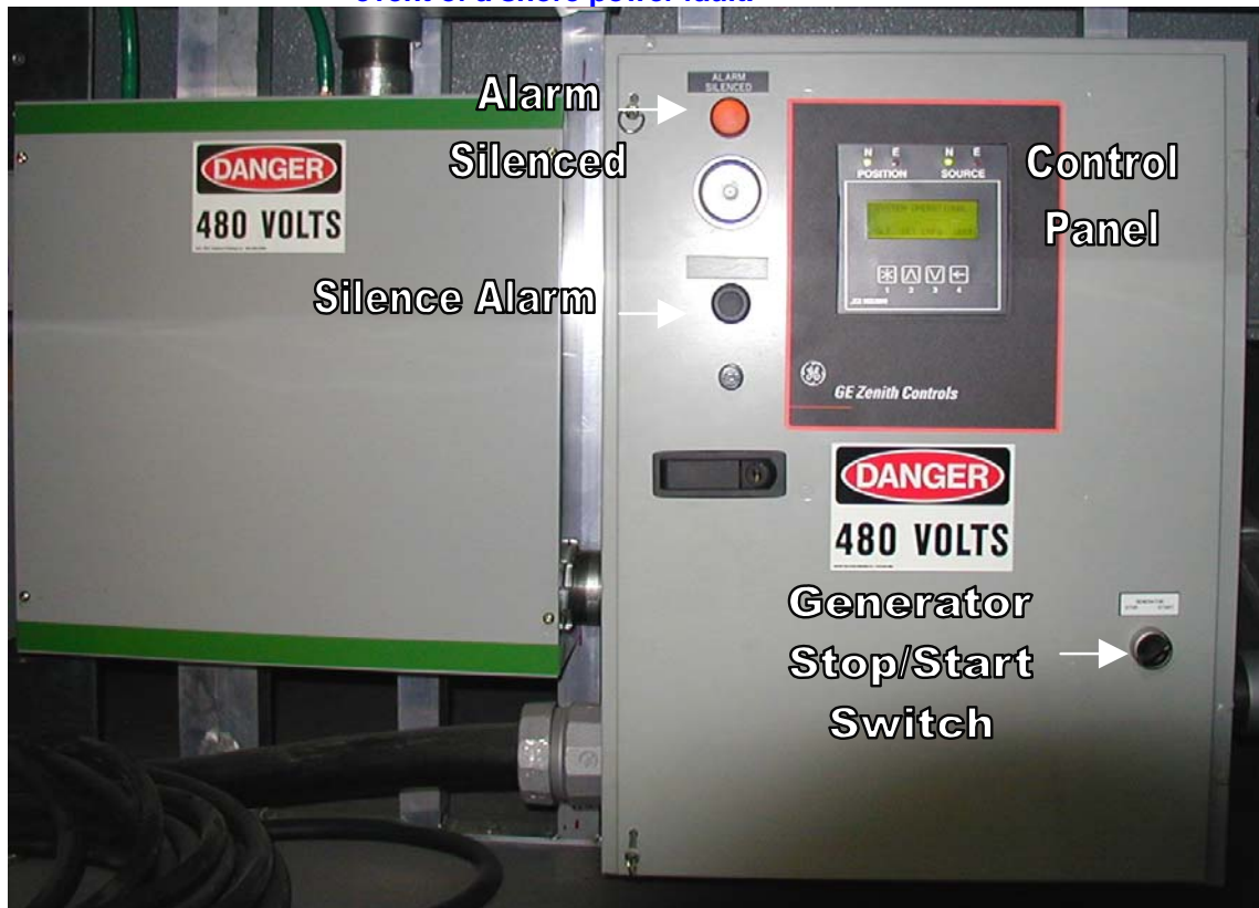
Figure 24: ATS Control Panel
