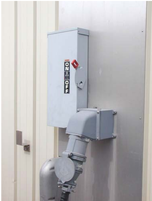
Figure 44: Shore Power Connection
