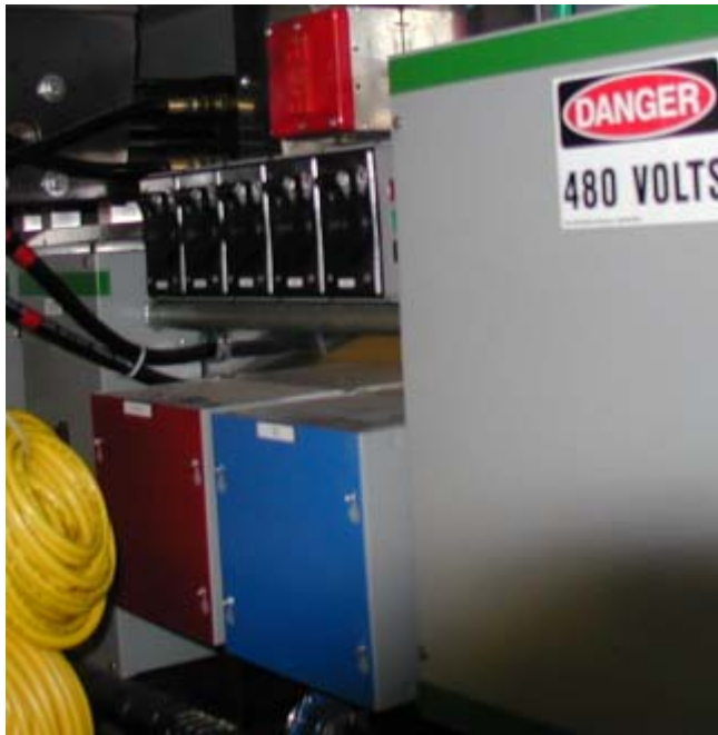
Figure 37: Fire Alarm and Code Blue Alarm Junction Boxes
