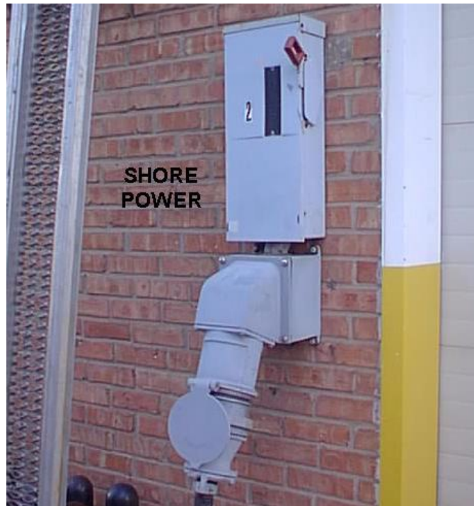
Figure 8: Shore Power Connection.
