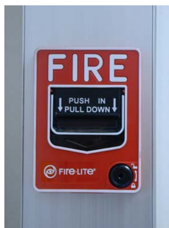
Figure 33: Fire Alarm Pull Station
