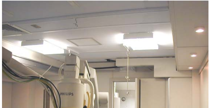
Figure 63: Procedure Room Lighting
